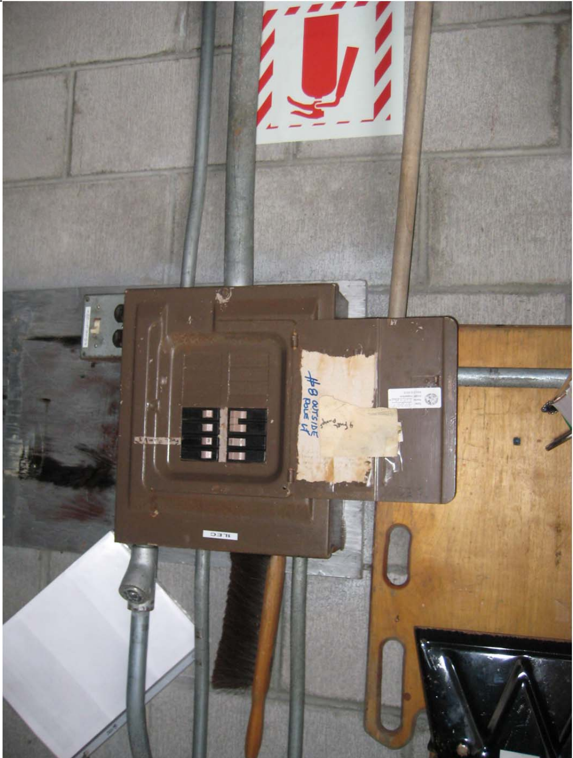
EE4 – Storage Room panel
